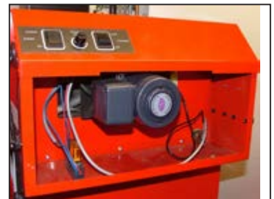
Figure 10-2: Boiler control panel (cover removed)
