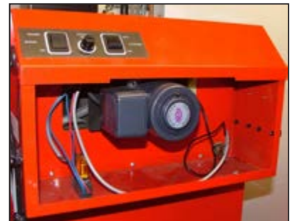
Figure 11-6: Boiler control panel (cover removed)
