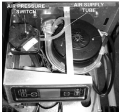
Figure 12-7: Air pressure switch and fan
