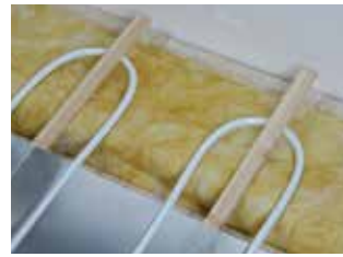
Notch or drill the joist to allow the pipe to pass through
